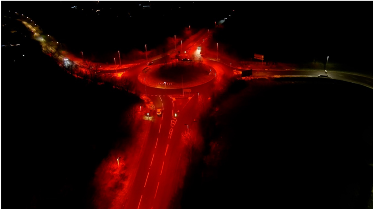
Photo 10: Red spectrum lighting install, A4440 Trotshill Way, Worcester.
